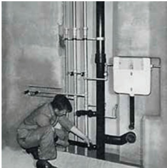
↑ Introducing the first concealed cistern in 1964
